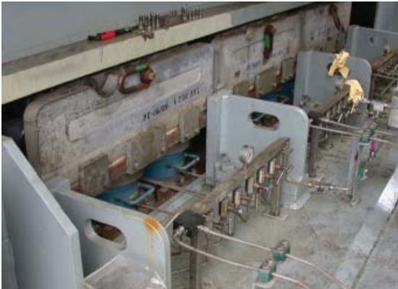
Above, one side of lift and roll system showing three 1250 ton capacity rollers resting on hydraulic rams.
