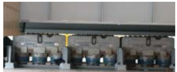
Profile view of hydraulic rams beneath the cantilever beams and Hilman Rollers.
